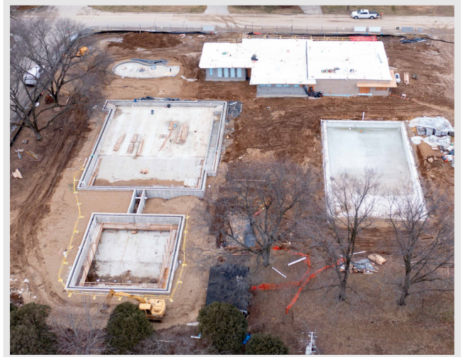
Above is a drone shot showing the completed concrete at all of the pool vessels as well the completed structure on the new pool house. What a transformation!
