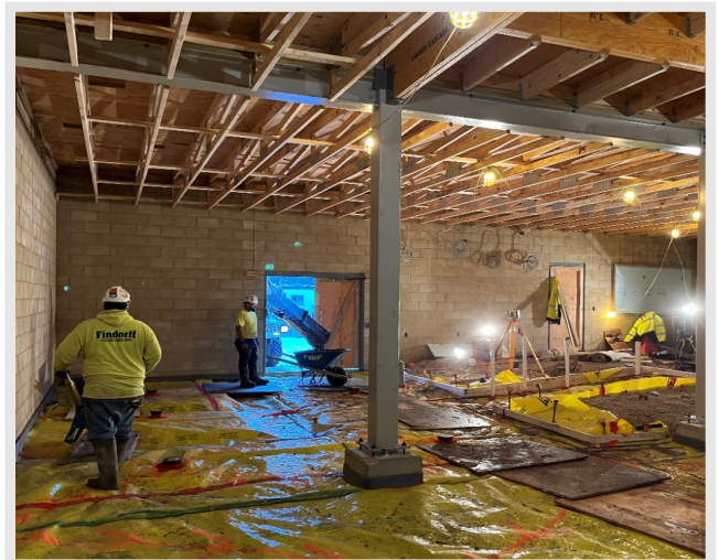
Below is a photo of the pool equipment room documenting the first concrete slab on grade pour of the project.
