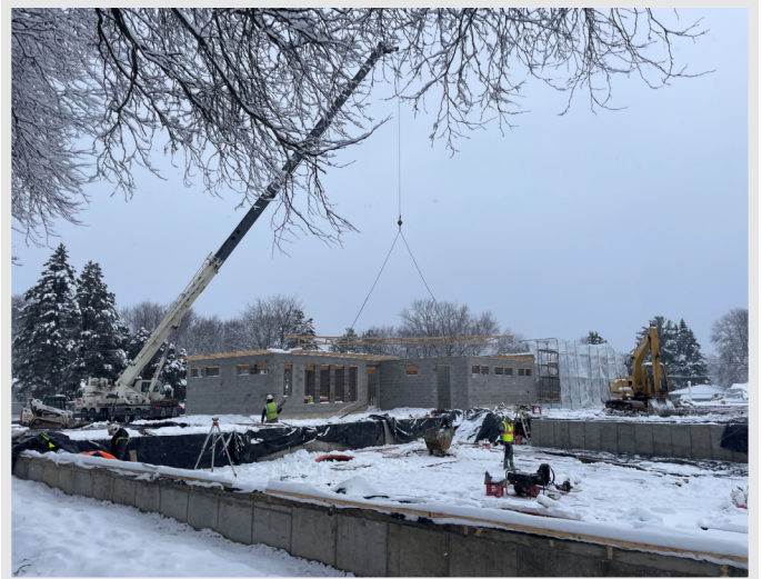
Below: A photo showing the completed concrete on the north walls of the competition/recreation pool. Crews are also shown laying out for the upcoming ramp and stair pours within the vessel.
