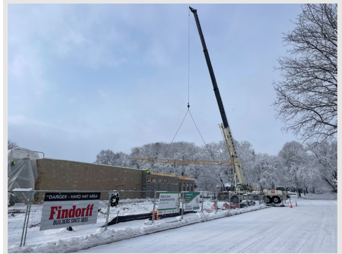
Above: A view from Barton Rd. showing one of the 54' wood trusses being set over the pool house locker rooms.
