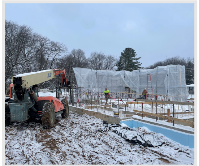
Below: Masons are mobilized and are setting up their scaffolding and winter protection.
