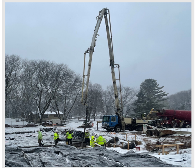
Above: A photo of the concrete pump truck that was used for the final concrete slab pour at the new competition/recreation pool.
