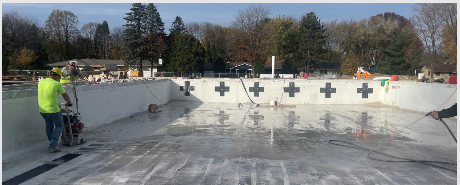
Above: A photo showing the scarfing process occurring at the existing lap pool that was described in this week's fun fact.
