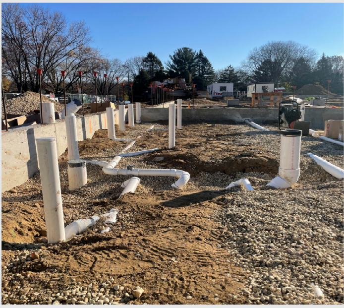
Above: Underground plumbing is underway at the new pool house. This means that the concrete floor slab is right around the corner!
