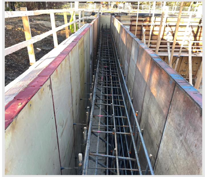
Above: Look at all of that reinforcing! This is a photo of the highwalls at the dive vessel. The tops of these walls will be over 24" thick to create space for the gutter that wraps the perimeter of the vessel.
