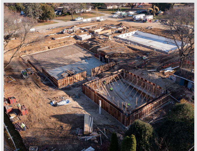
Below: A view from the southwest corner of the site showing a better look at the new dive well and competition/recreation pool.
