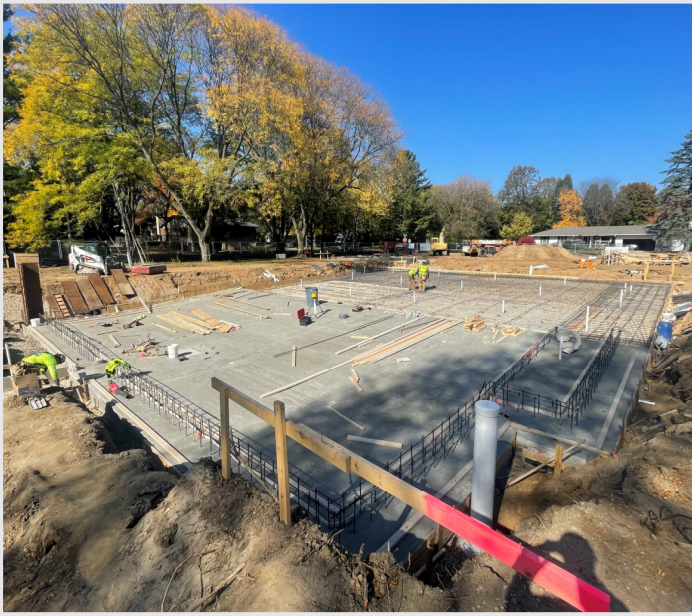
Above: The first half of the new competition/recreation pool has been poured. After the north half is poured, wall forming and reinforcing will kick off.
