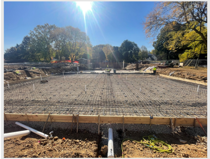
Above: Reinforcing at the north half of the new competition/recreation pool is complete and ready for the pour.
