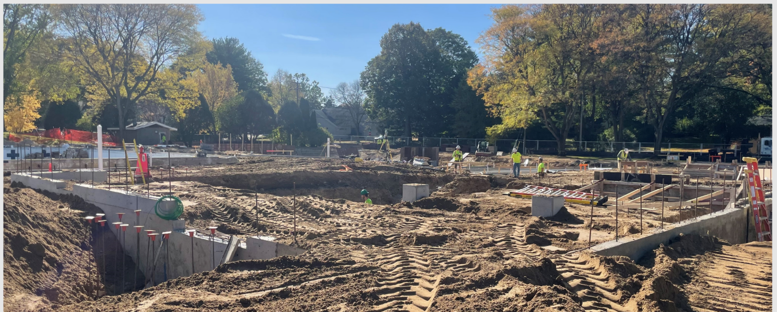
Above: A photo taken from the northeast corner of the new pool house showing the progress the teams have made on the footings and foundations over the last two weeks.
