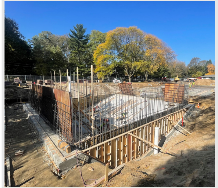
Above: Forming and reinforcing for the low walls at the new dive well is nearly complete and will be poured early next week.
