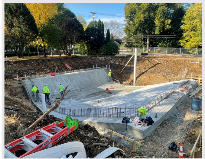
Below: The concrete base for the new dive well has been poured and wall reinforcing is well underway.
