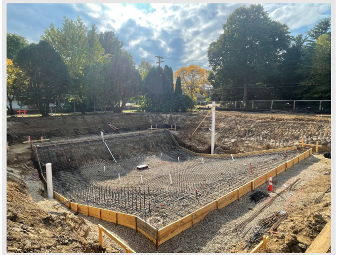
Above: Reinforcing at the slab of the new dive well is nearly complete and the concrete slab pour will soon follow.
