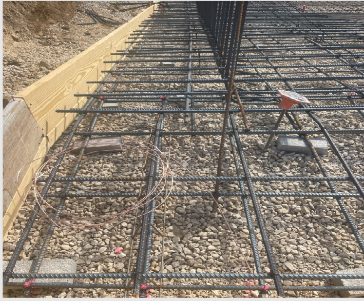
Above: A photo showing what the grounding, that was mentioned in the fun fact, looks like. Look closely for the wire and its connection to the rebar.
