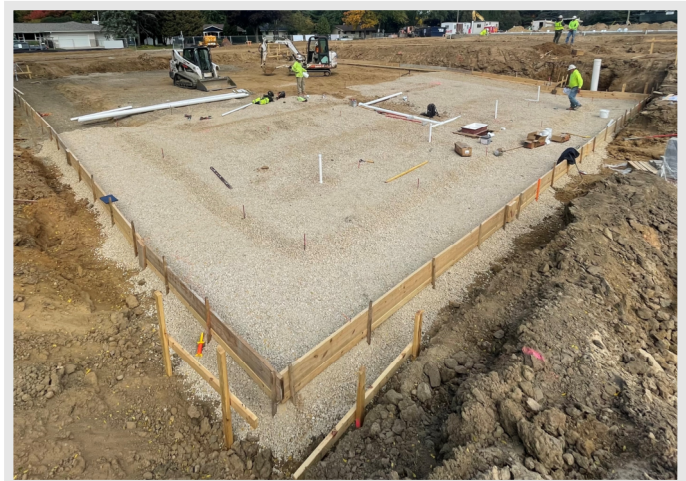
Below: Stone subbase and under pool piping is well underway at the new lap pool and reinforcing will be starting next week.
