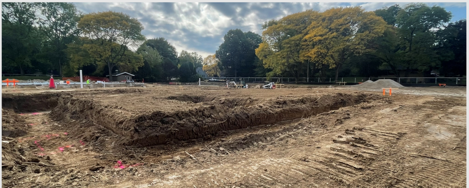
Above: A photo showing the start of the excavations for the new pool house. Footings and foundations will start next week!
