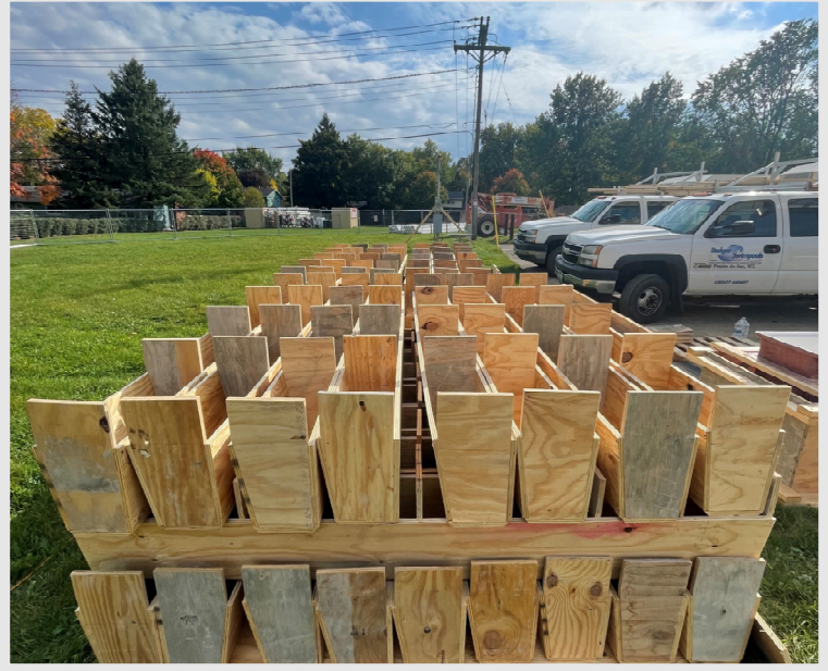
Above: Crews have already started prefabbing the forms for the pool gutters that exist at the top of the pool walls. They'll prefab these forms to stay ahead and efficient when it comes time for the pour.
