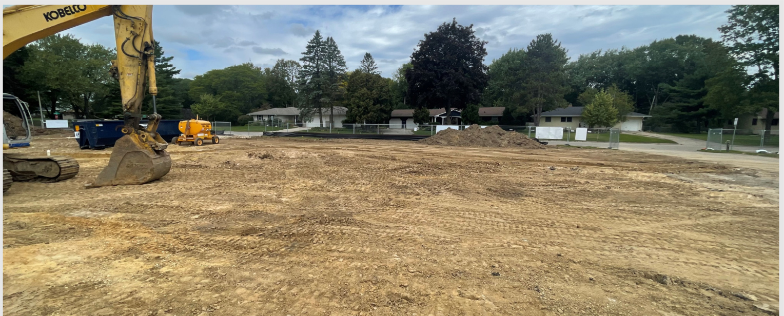
Above: You guessed it right... This is a photo showing exactly where the old pool house used to exist. Keep an eye out in the coming weeks as the footings and foundations will soon be started, and the footprint of the new pool house will begin take shape!
