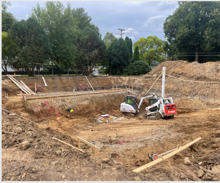
Above: The dive vessel excavation is complete, pool piping is in progress, and the pool base and walls will soon be following!
