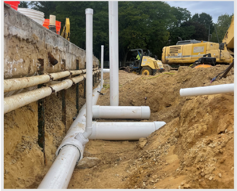
Above: A progress photo showing the new pool piping at the existing lap pool that is currently being refurbished. This new piping will soon serve the new surge tank.
