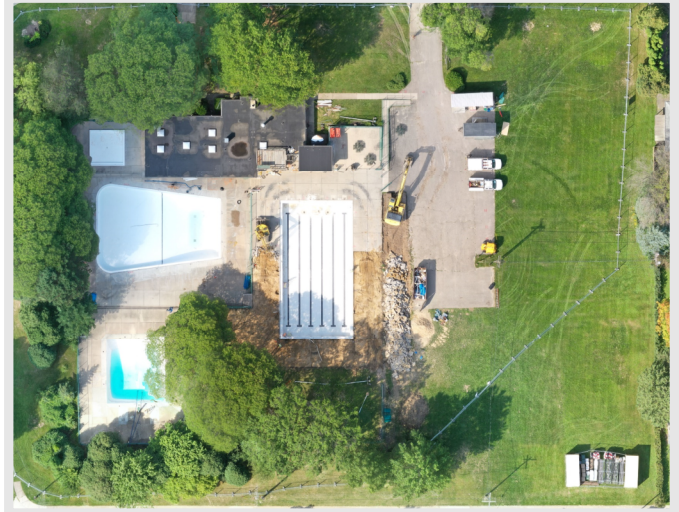
Above: Photo was taken on 9/7/2022, which was just a day after teams officially mobilized on-site and prepared for construction.
